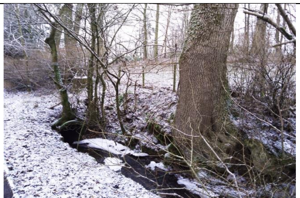
North-east end of culvert on Castlestanes corner, mature ash on west side of burn. 54
